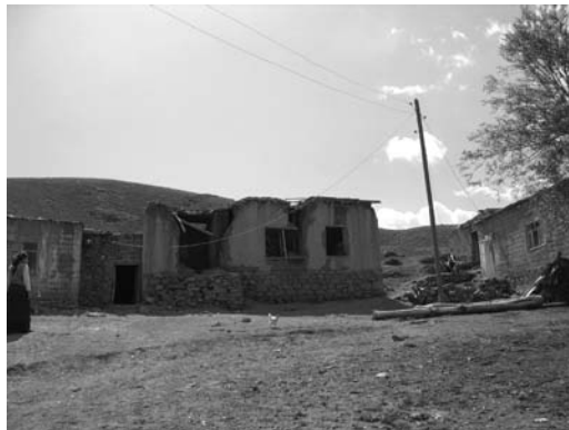
Ruined Buildings in Taşnacak, July 2006
